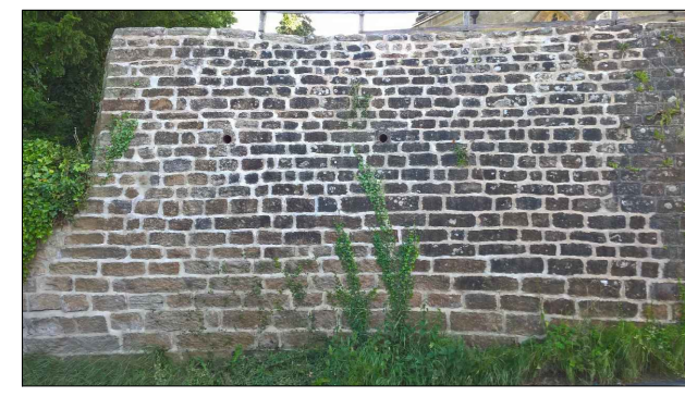
BOUNDARY WALL - BEFORE COLLAPSE
