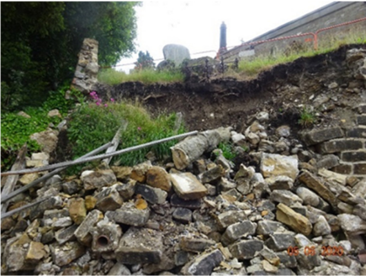
Collapsed section to north corner
